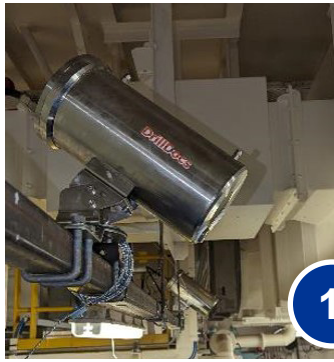
Explosion proof cameras mounted in the shaker room.
